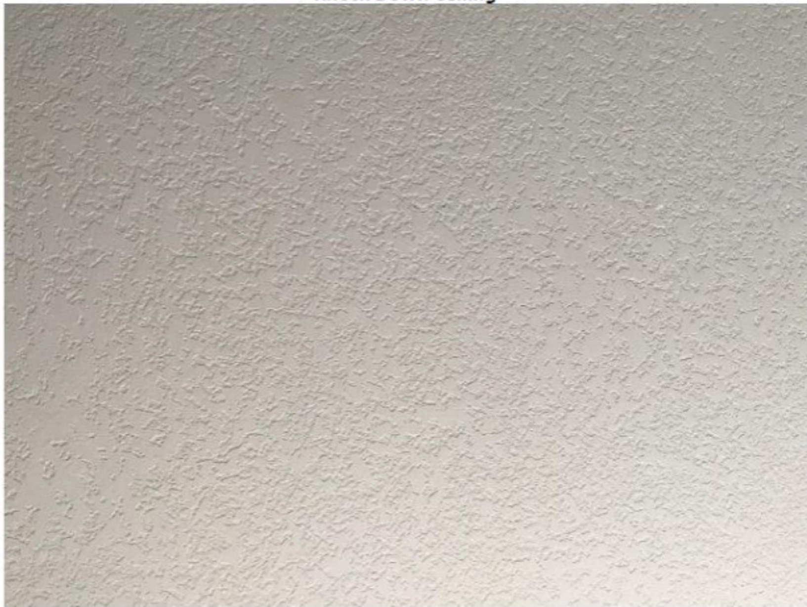
Knock Down Ceiling
